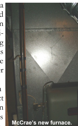
McCrae's new furnace.
